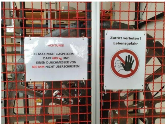
Schutzgitter am Coiltower
