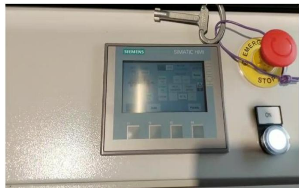
Control display, start button and emergency stop switch
