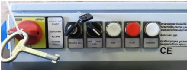
Electric cabinet with operating buttons
